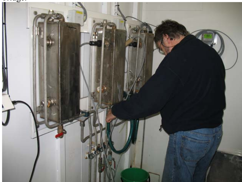
Figure 10. Water sampling from units leading water from two fish wells and outside water into a central monitoring and sampling unit onboard a well boat designed for closed transport. Photo: Trond Rosten
